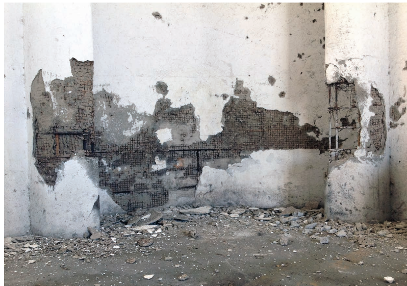
Figure 16. The Magliana warehouse walls before the restoration works, 2012, © Sixxi
