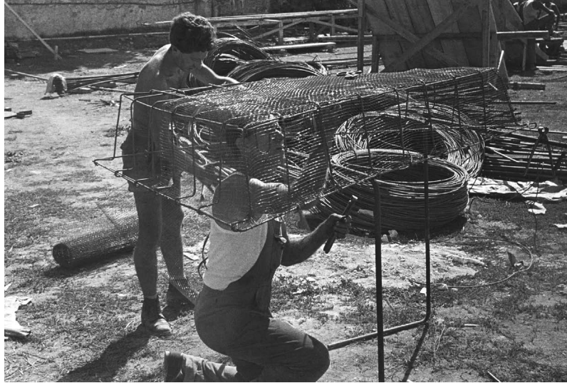
Figure 9. Workers creating one of the 1620 inner steel weaves of the ferroconcrete tavellone for the dome of the Palazzetto dello Sport, 1956 (reproduced by agreement of Centro Archivi Maxxi, Rome)
