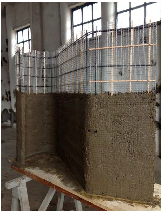
Fig. 5. Full size model of a portion of the Magliana Warehouse's curly wall, 2013 (Photo Sergio Poretti, SIXXI Project).
