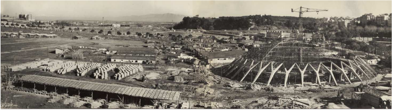
Figure 17. The Palazzetto dello Sport full worksite: on the left, the prefabrication site; on the right, the cast-on-site and assembly site, 1956
